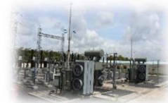
Huu Thanh Phase 1: 63MVA (Total 189MVA)
