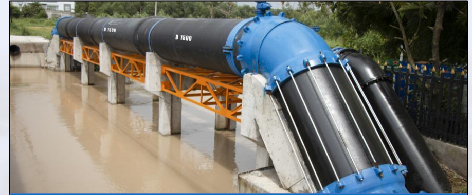
RAW WATER TRANSMISSION PIPE D1500 BINH DUONG
